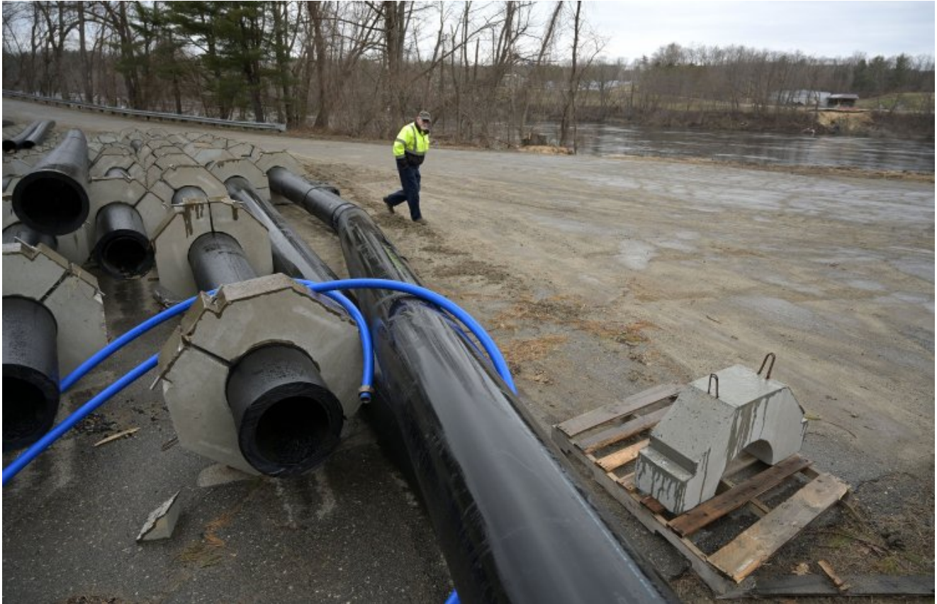
Winslow Public Works Director Paul Fongemie walks past 16-inch sewer line on April 10 at the Chaffee Brook Pump Station in Winslow. The pipe will replace the existing line that runs beneath the Kennebec River to Waterville's Kennebec Sanitary Treatment District. Rich Abrahamson/Morning Sentinel file Buy Image
